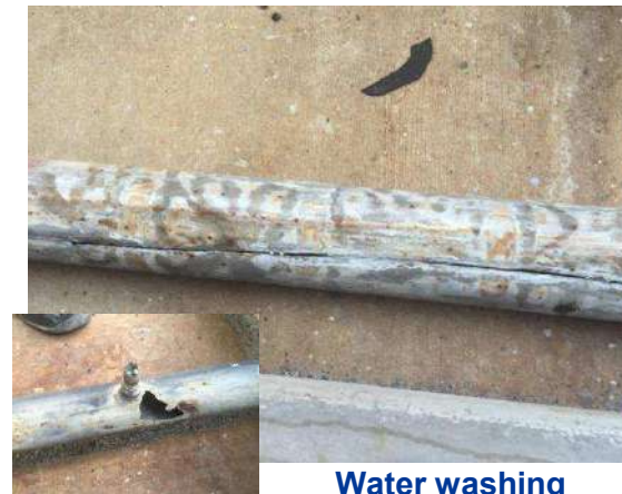
Wear damage of carbon steel tube.
